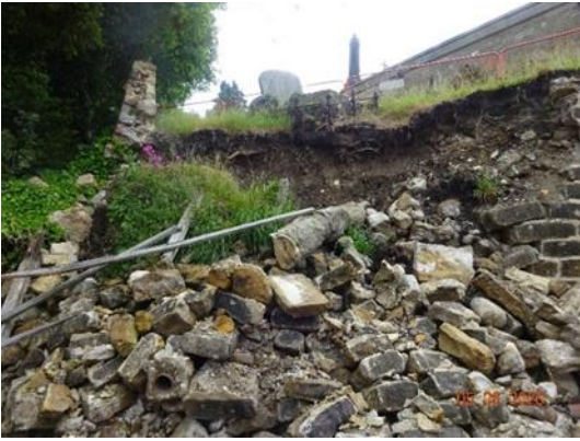
Collapsed section to north corner
